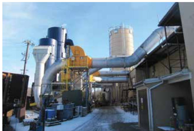
Pressure relief system panels around the top of a silo can help alleviate pressure and avoid combustible dust explosions.
