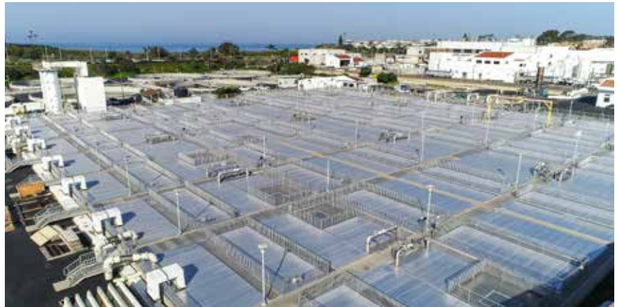
Installing new, flat covers at the Encina Wastewater Authority, in Carlsbad, Calif., provided benefits related to safety, odor control, and aesthetics. CST
