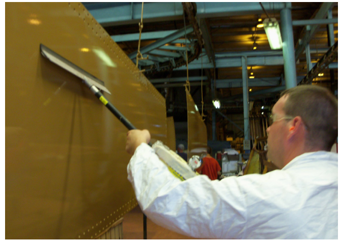
All tank coatings should be tested for quality assurance.
