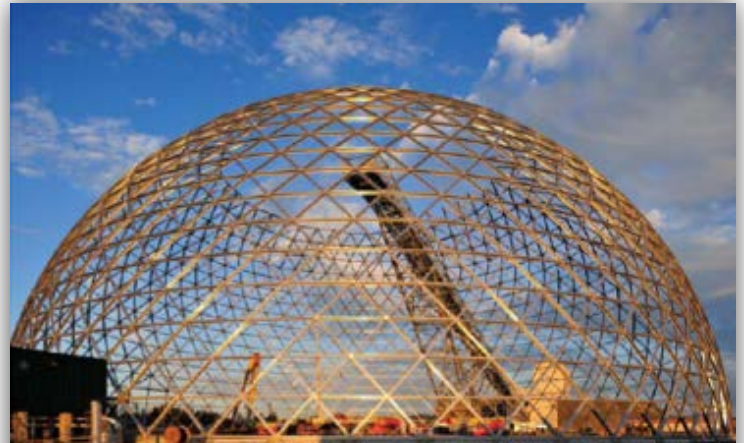
In total, 3,363 beams were constructed into aluminum gussets to form the structure. Photo courtesy Detour Corporation and Graeme Oxbly.
