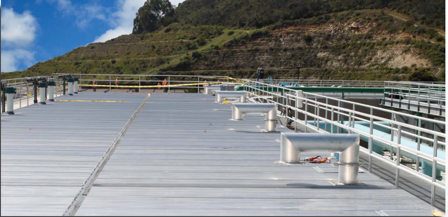
Twin Oaks Valley WWTP San Marcos, California - 30' x 165'
