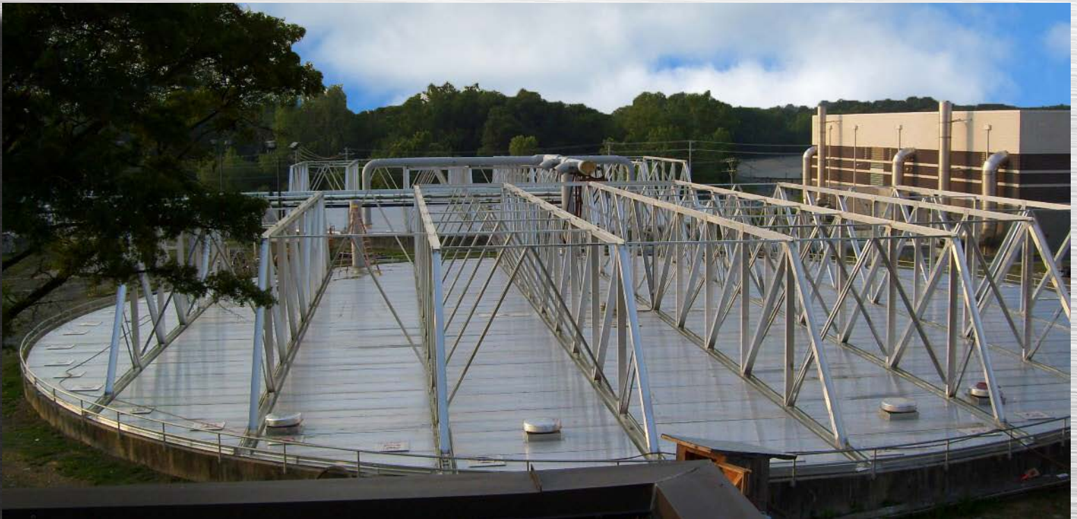
McAlpine Creek WWMF, Charlotte, North Carolina - (2) 130' diameter
