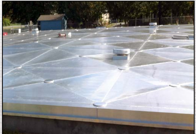
Thomasville NC Water Department Thomasville, North Carolina - 85' x 126'
