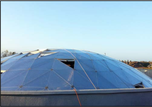
Port Arthur Water Treatment Plant Port Arthur, Texas - 202' diameter
